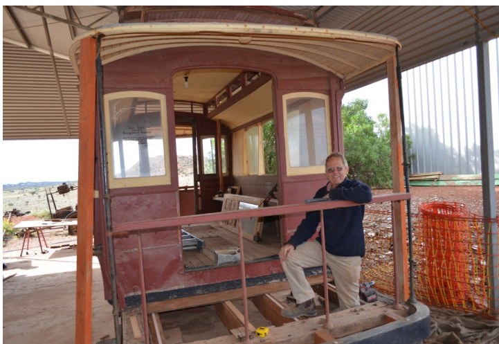
Stephen Peacock in the process of redoing the floorboards on the platform.
