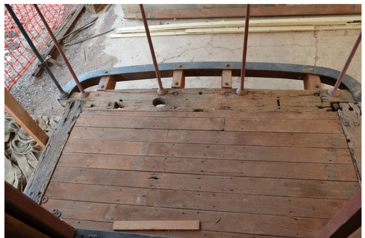
The floorboards replaced on the platform and awaiting new metal front cover.
